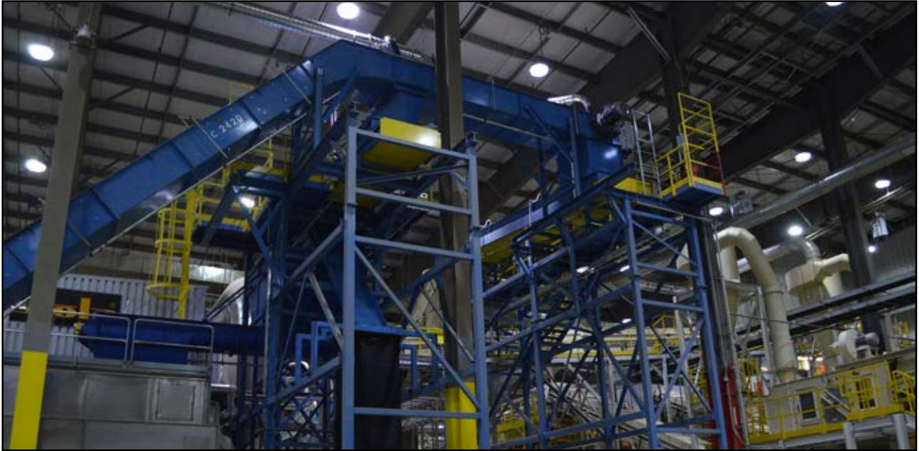
Edmonton, Canada Drying Plant
