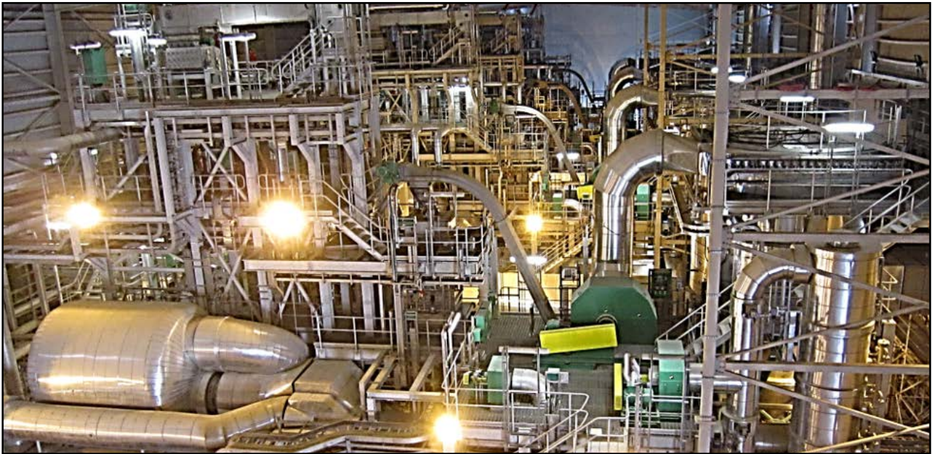
Doha, Qatar Drying Plant
